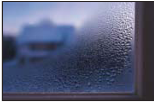
Condensation on the inside of a windowpane.
